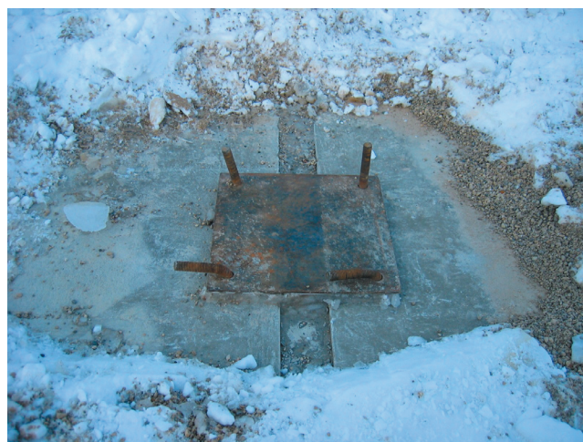
Figure 2.3. Anchor rods run over by crane.
